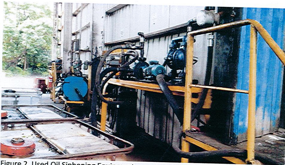
Figure 2. Used Oil Siphoning Equipment
